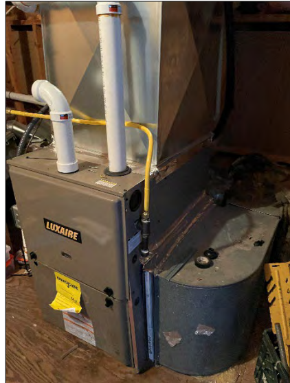
View of mechanical area located at 84 Cannifton Road N.
